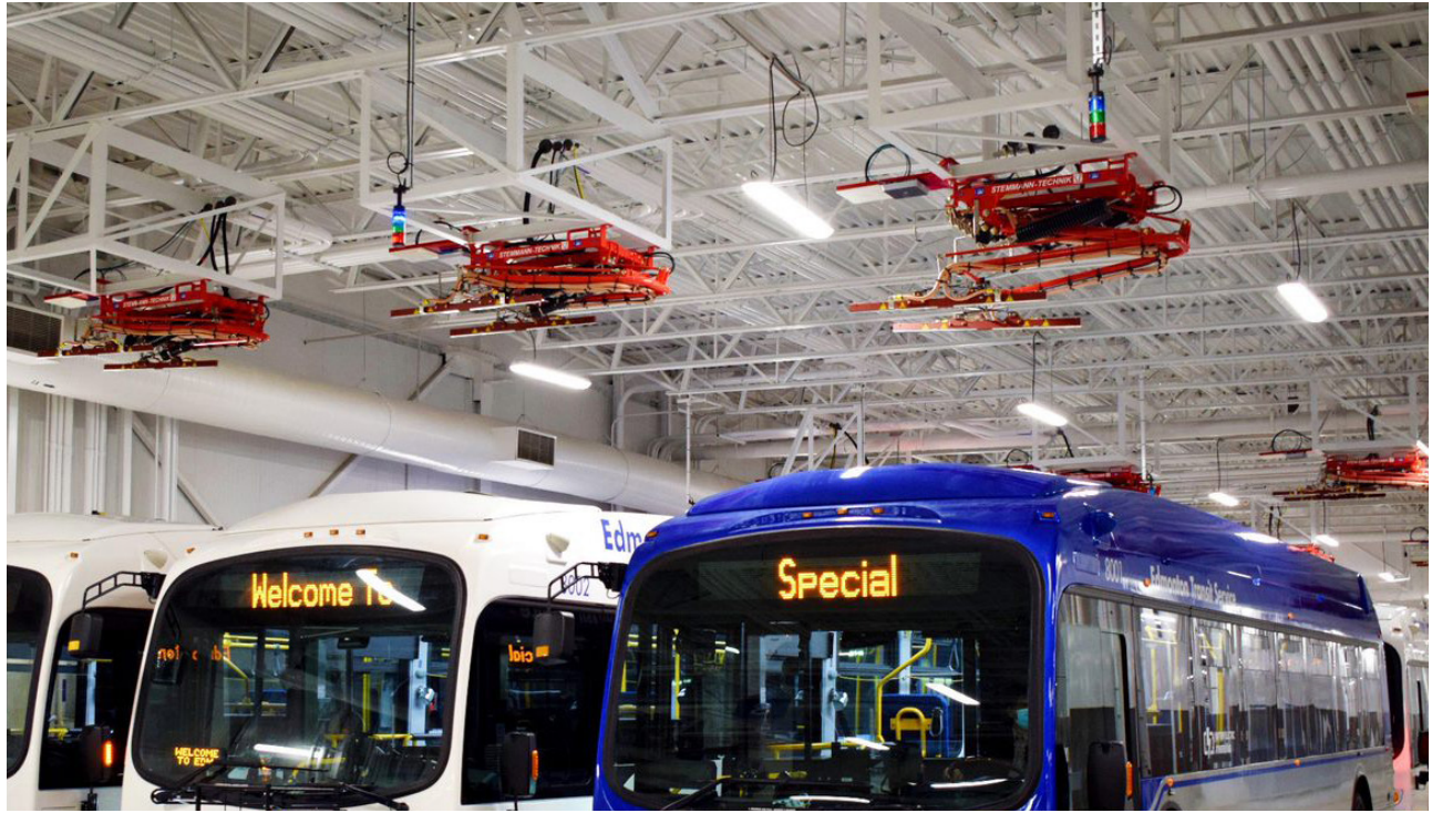
Figure 9: Edmonton Transit Service collaborated with Proterra Energy™ to install 26 ABB HVC 150 kw pantograph chargers using RFID technology as guidance systems. Pantograph chargers create a future-proof transit facility enabling bus automation solutions. Image credit: Proterra
